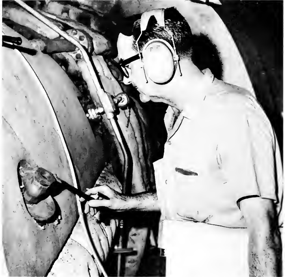
Ear muffs protect the hearing of Robert J. Roy, shift engineer on watch at the Miraflores Substation, shown checking one of the gas turbo-generators by making a flame inspection. Roy is inside the protective aluminum covering of the generator standing next to the generator itself. The asbestos padding over the turbine is a protection against heat.
